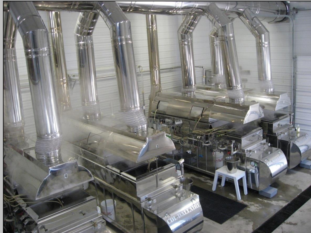
Maple Processing Research Facility (MPRF) at UVM PMRC
